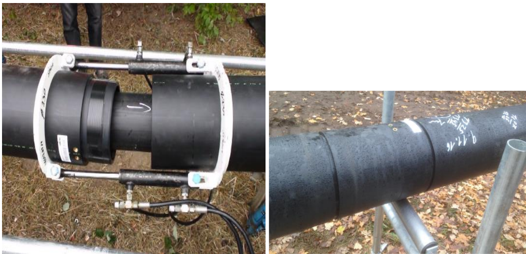
Fig. 1.5: Step 3a – Joining the cable carrier-pipe long-shots embedding the internal cable using the SIMOFUSE® process at the Stade test and pilot site
