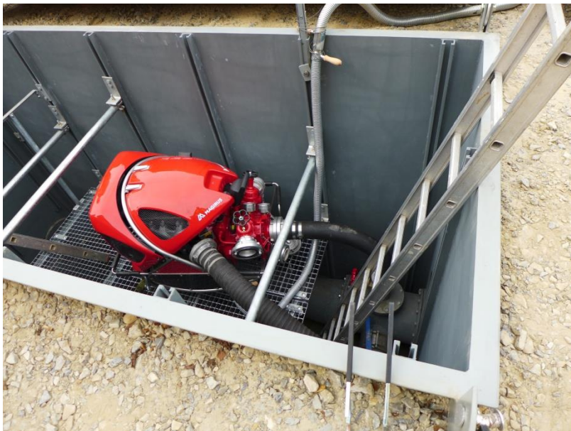
Fig. 3: AGS test operation at the Stade test and pilot site ©
